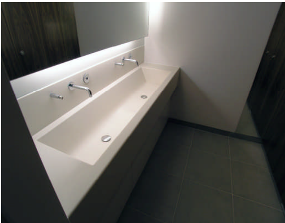
Offices Pall Mall Levada trough in Corian
