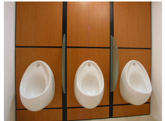
Cherry laminate urinal ducts with toughened glass dividers
