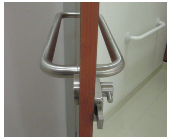
Ambulant disabled cubicle with back to back stainless steel pull handles
