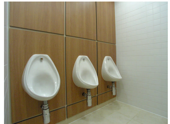
Urinal duct panels in Verona Walnut
